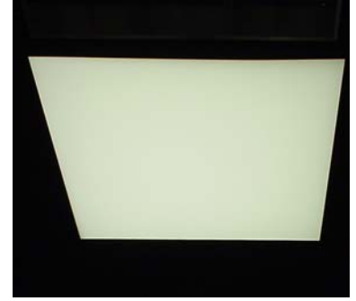
Installed Troffer Illuminated
